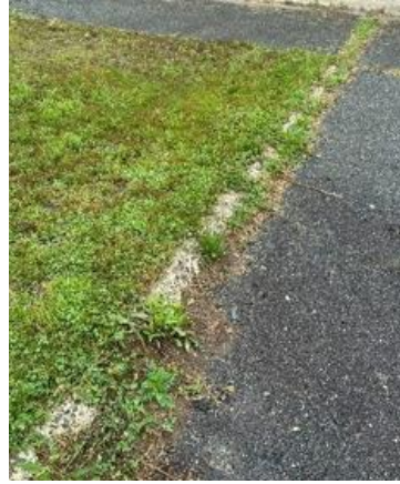
Deteriorated concrete curb
