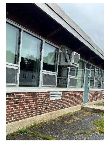
Window-Mounted AC Units
