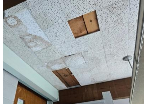
Ceiling Water Damage
