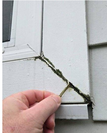
Window Sealant Failure
