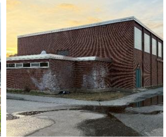
Efflorescence at masonry
