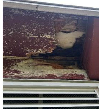
Deterioration of Plywood Soffit and Frieze
