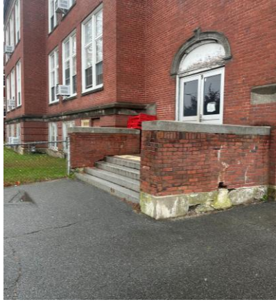
Spalled Concrete at Entry
